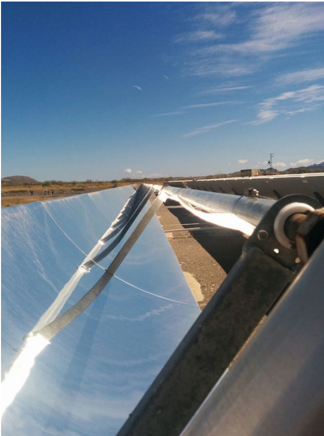
Figure 4 - Assessment of insulating strips under concentrated solar radiation
