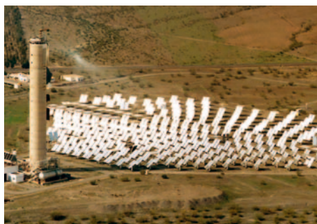
(b) 7 MW th solar tower, PSA, Almería, Spain (CESA 1)
